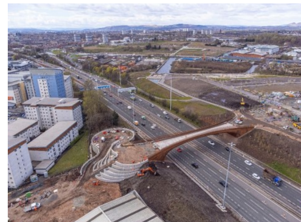
Fig 4.c.1 - Sighthill pedestrian and cycle bridge: under construction, April 2022. This photograph is the property and copyright of BAM Nuttall Limited.
