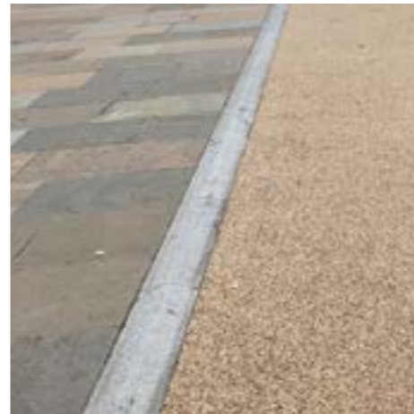
MTL-04 Marshall's segregation kerb Between cycleway and footway
