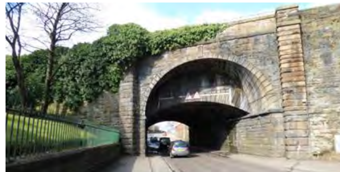
Figure 4.7: Width constriction due to aquaduct crossing over Maryhill Road.
