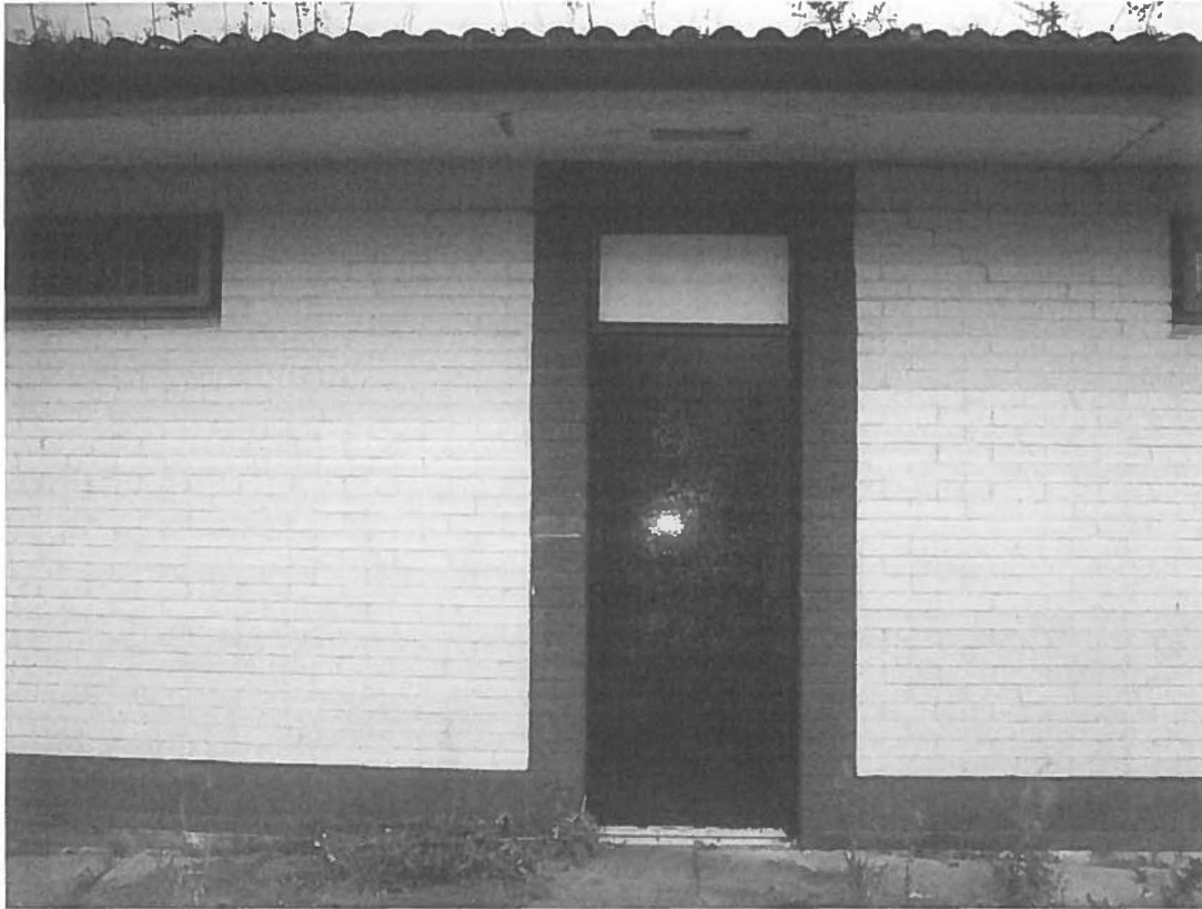
9. CRACKING TO BRICKWORK TO EAST ELEVATION OF GAMES HALL
