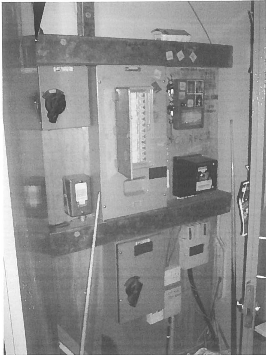
15. ELECTRICAL SWITCH GEAR AND METER
