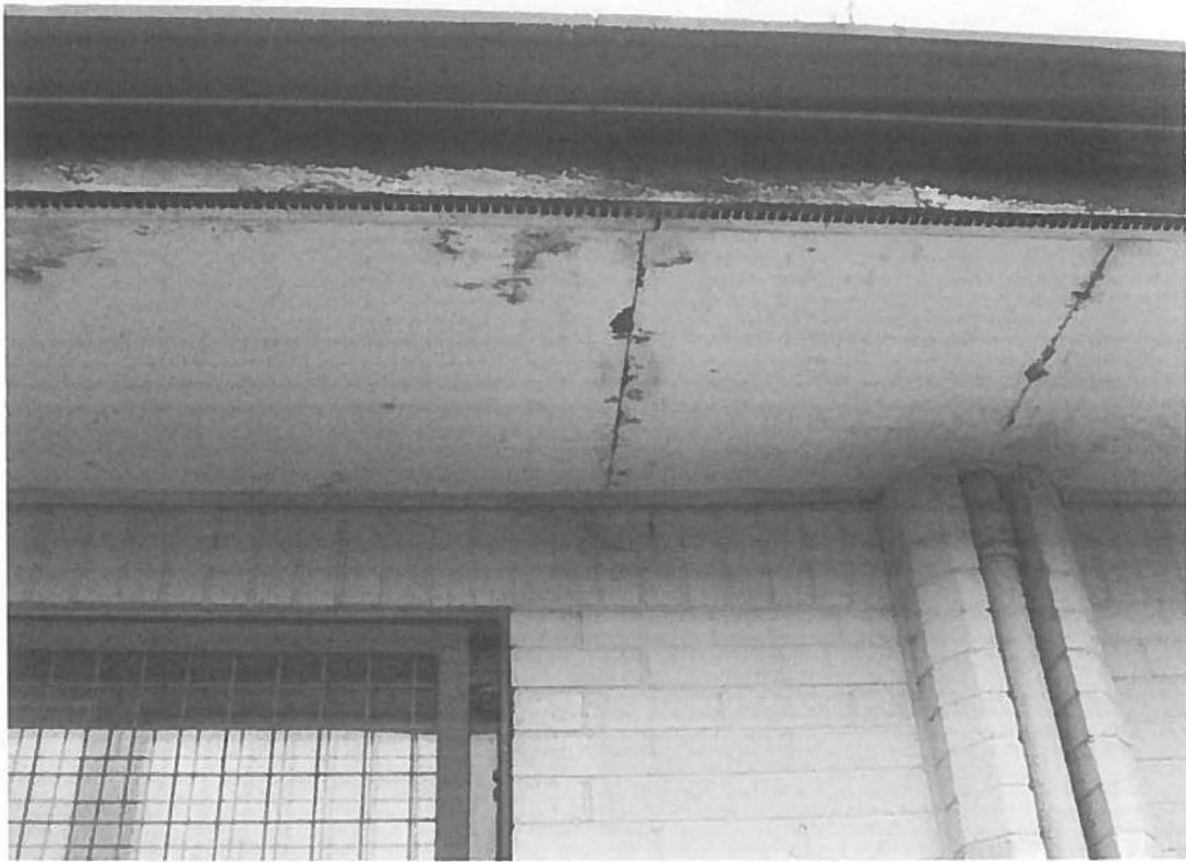
7. WATER DAMAGE TO SOFFIT BOARDS
