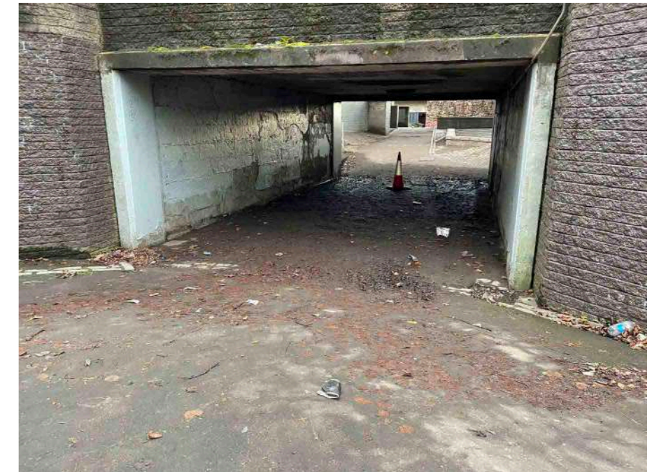
Uninviting underpass with severe drainage issues preventing access.
