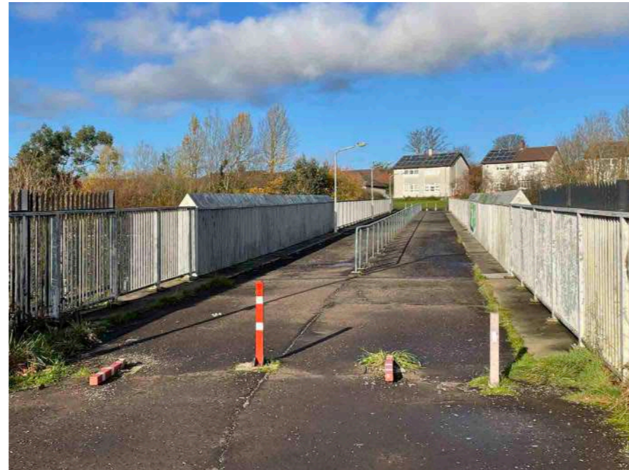
The Robroyston Road - Winifred Street bridge has potential for public realm improvements.
