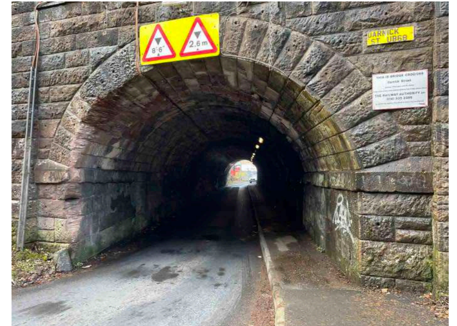
The 'blind tunnel' on Darnick Street is extremely constrained and uncomfortable to use.
