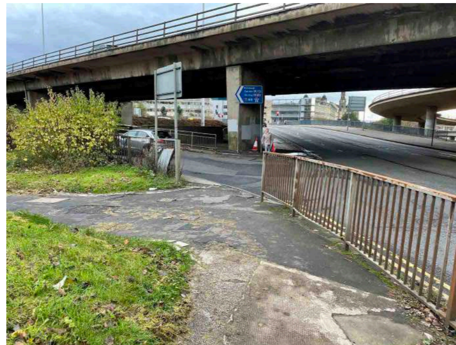
Lack of crossing infrastructure and poor pedestrian and cycle environment on Castle Street.
