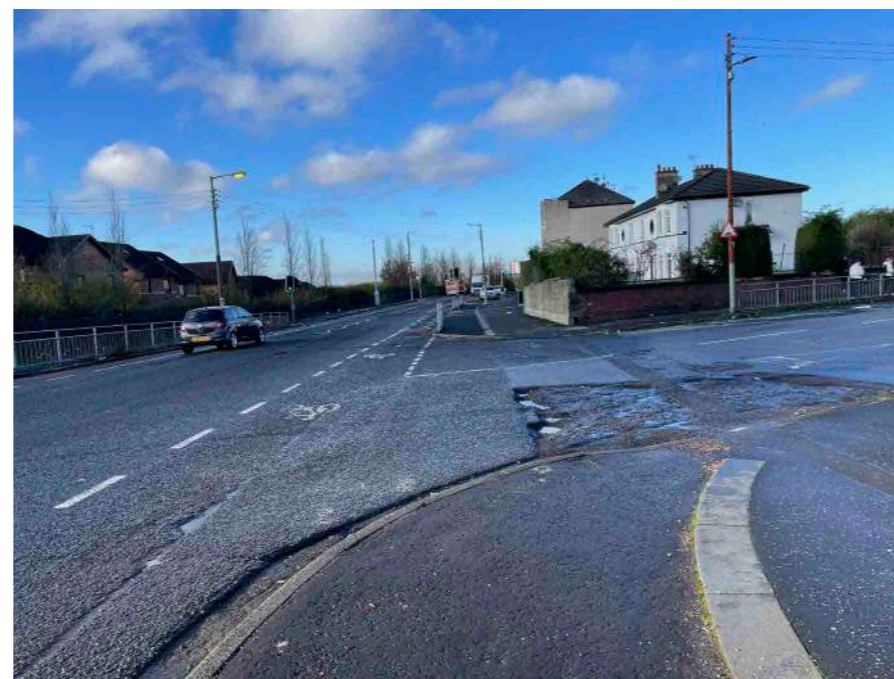
Poor quality surfaces, wide side road junction and large corner radii on Provanmill Road/Langdale Street (Blackhill).
