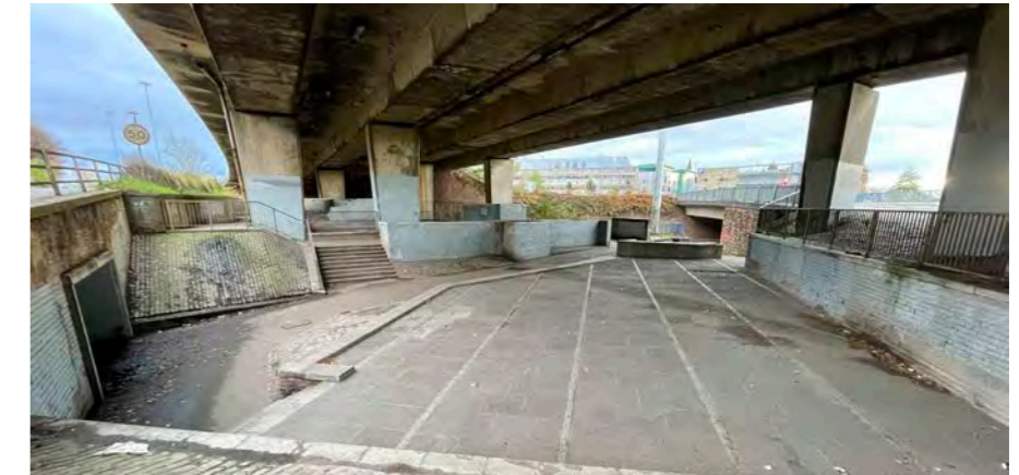
Castle Street Plaza fails as a welcoming and active thoroughfare.
