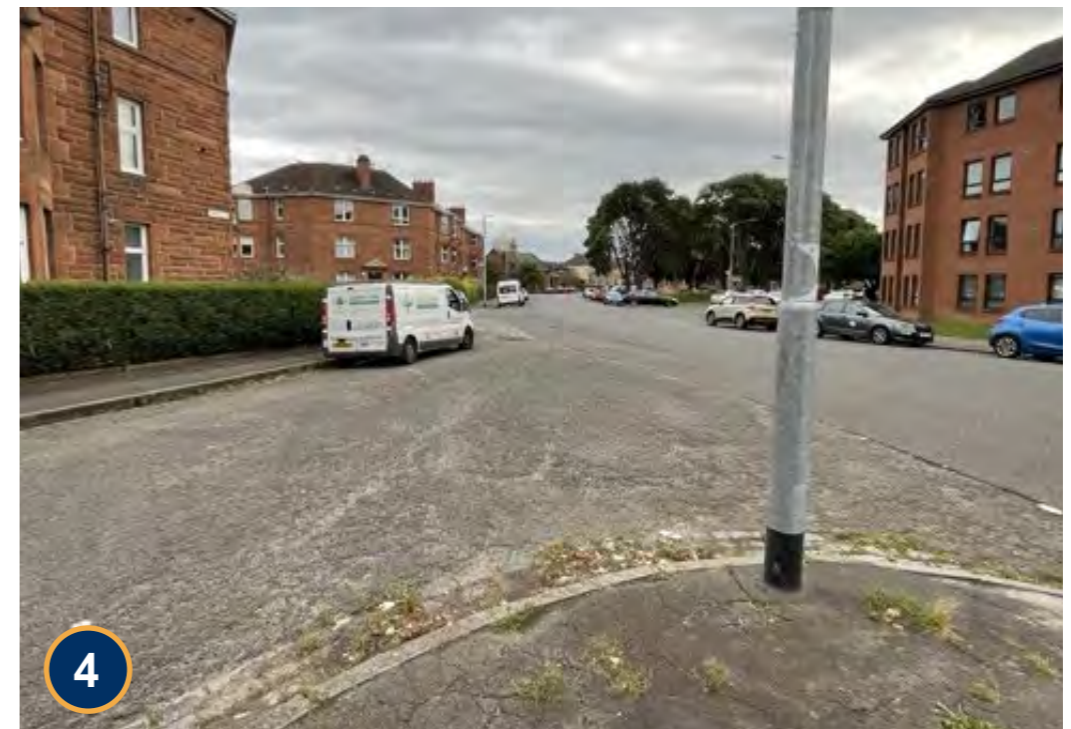
4 Generally dangerous and inaccessible crossing arrangements.
